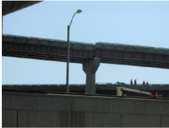
Figure 2. Bridge in New York that has fallen off its bearing and come to rest on the pier cap.
