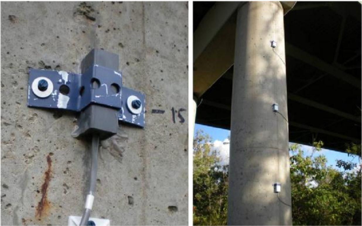
Figure 25. Sensors mounted on bridge: individual sensor (left) and a three sensor array (right).
