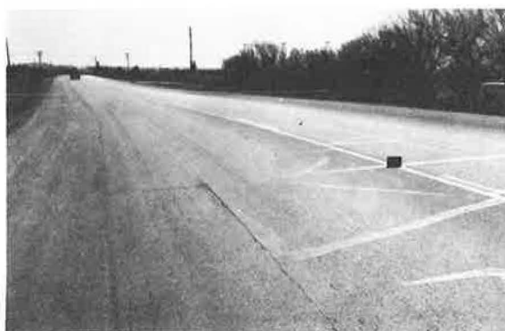
Figure 18. Progression of a particular cracking pattern through March 1959.
