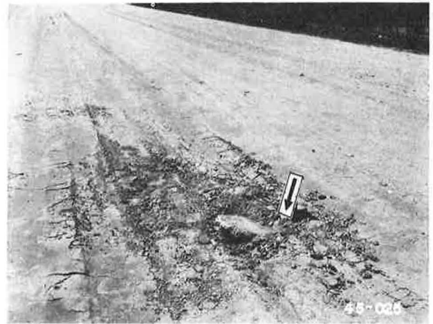
Figure 10. A condition indicating improper seating was found here.
