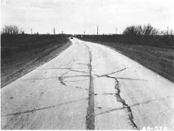
Figure 2. Original pavement condition before overlay of HMAC surface.
