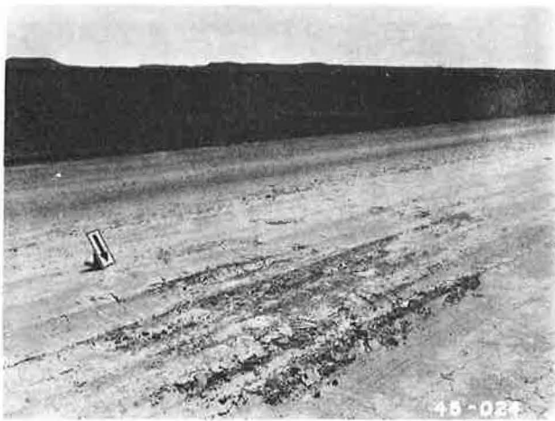
Figure 11. A condition indicating improper seating was found here.
