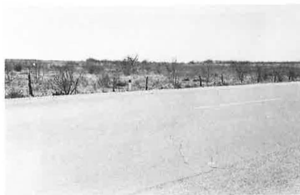
Figure 22. A typical failure pattern on design section No. 2 in 1959.
