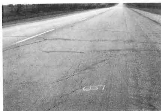
Figure 24. A typical failure condition showing distress of design section No. 2 in 1964.
