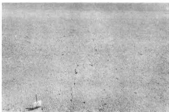
Figure 19. First sign of distress on design section No. 3.
