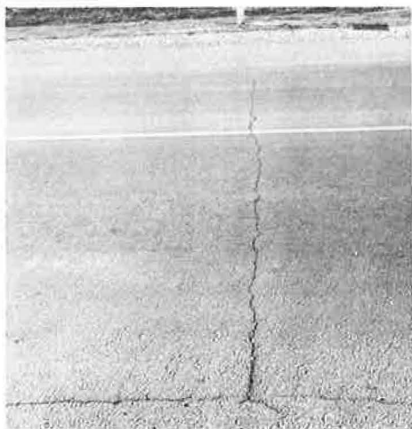
Figure 15. Progression of a particular cracking pattern through March 1959.
