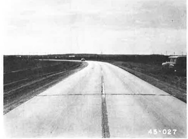
Figure 3. Original pavement condition before overlay of HMAC surface.
