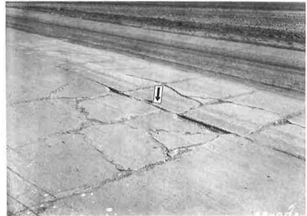
Figure 5. Original pavement condition before it was broken up and recompactd.
