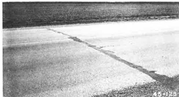
Figure 16. Progression of a particular cracking pattern through March 1959.
