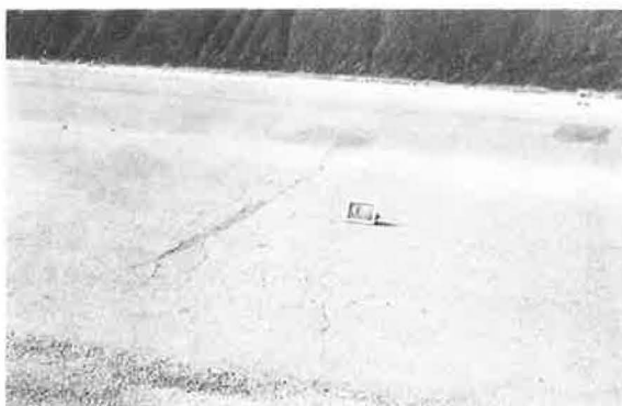
Figure 20. A typical failure pattern on design section No. 3, in 1961.
