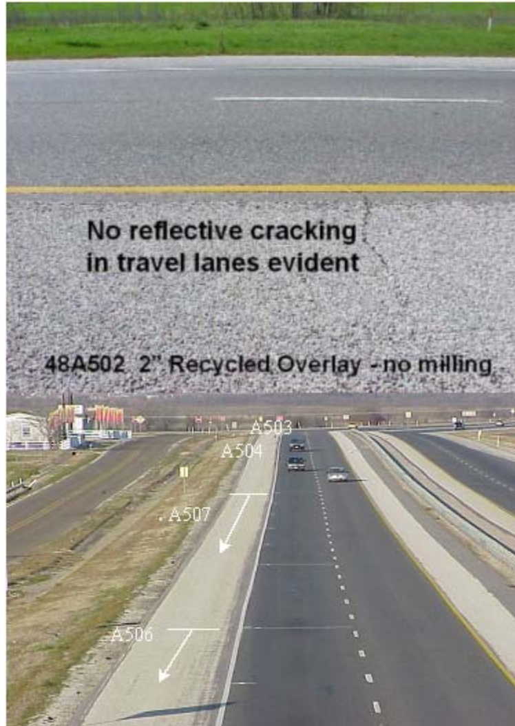
FIGURE 2 Current pavement conditions on SPS-5 section (US-175).
