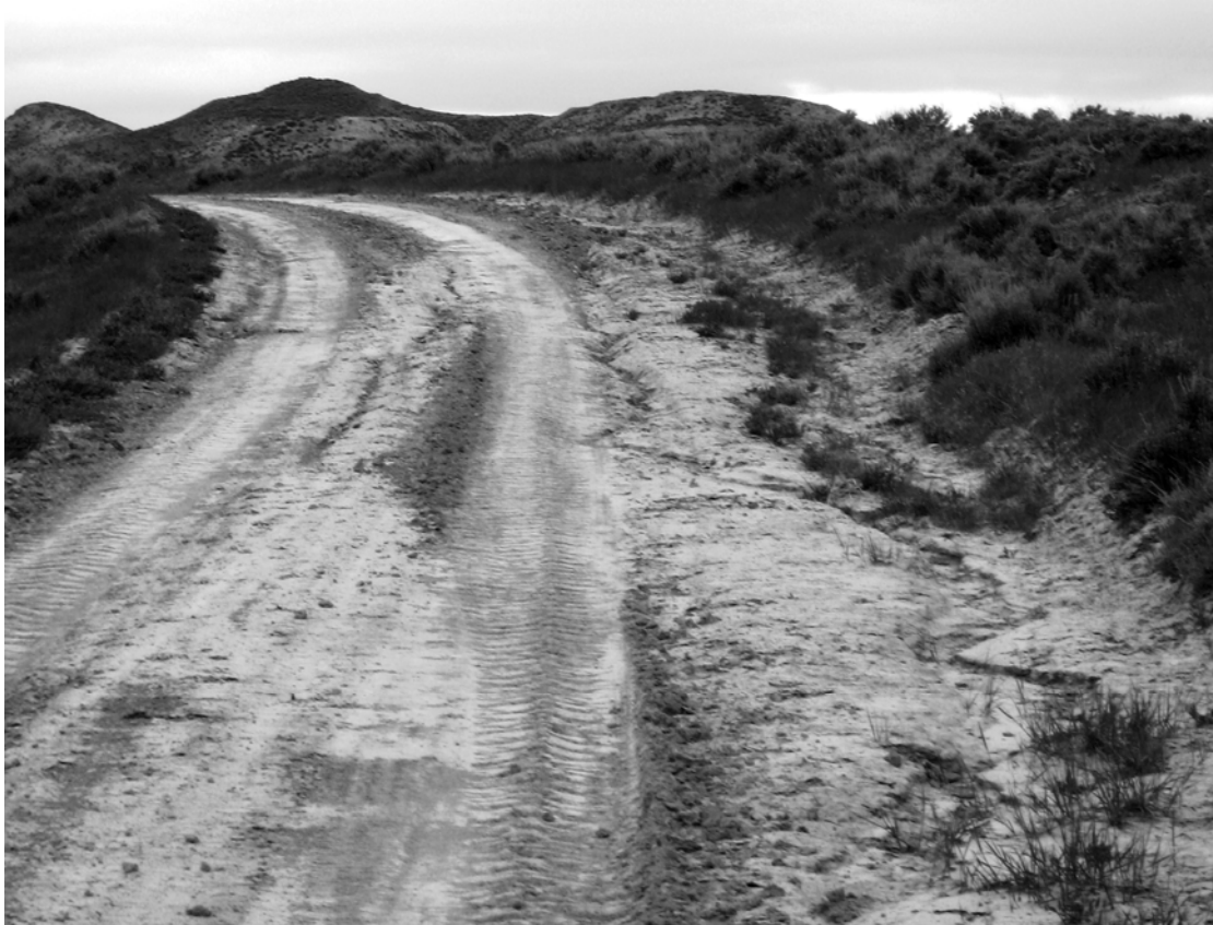
FIGURE 3 County road with small gully in secondary ditch, channeled into main ditch after a recent, heavy rain.
