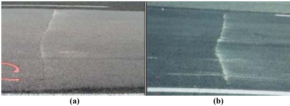
FIGURE 7 Crack developments on remixer section (US-84): (a) before remixer process (US-84) and (b) 2 months after remixer process (US-84).
