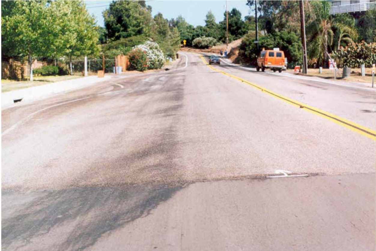
FIGURE 4 Effects of a rain storm that occurred within 24 h after chip sealing.
