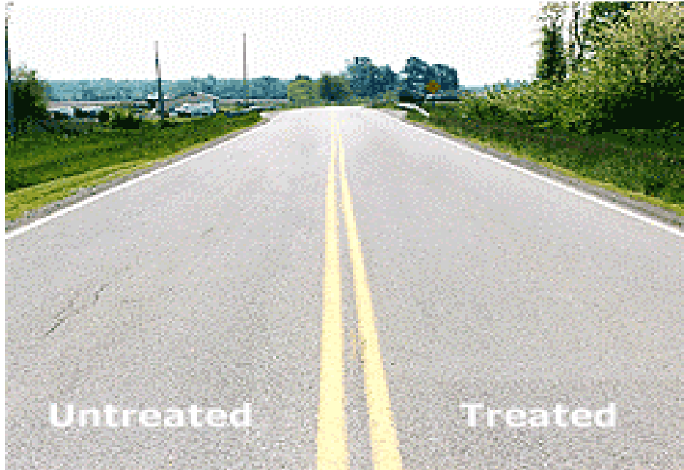
FIGURE 6 Logan County Road 154 in Ohio in July 1999, 24 months after treatment.
