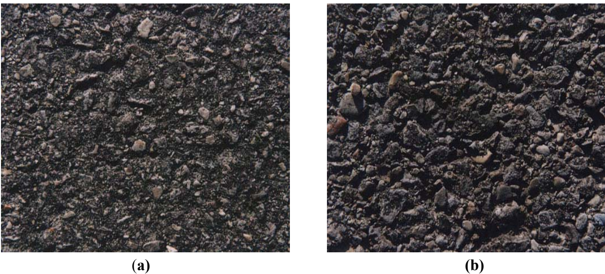
FIGURE 5 Logan County Road 154 in Ohio in September 1998, 14 months after treatment: (a) treated surface and (b) untreated surface.
