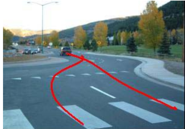
Figure 3 - Insufficient Entry Path Curvature (This layout also suffers from entry path overlap)
