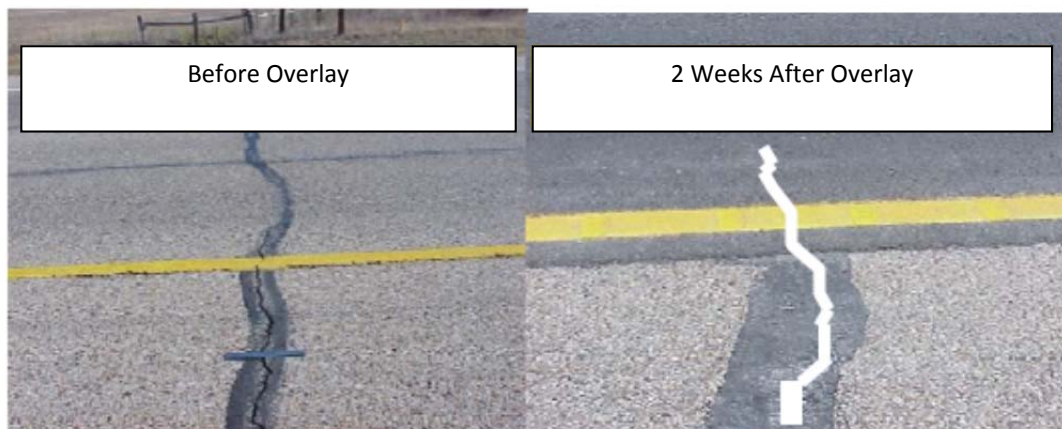
FIGURE 8 Reflective cracking on US-175 remixer section.
