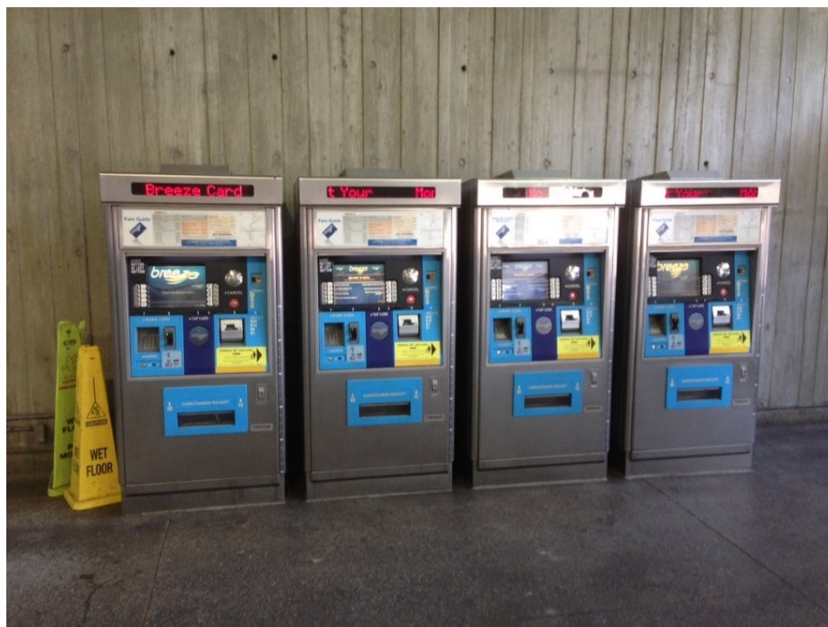
FIGURE 4 Four Breeze ticket vending machines in MARTA Midtown Station. The same equipment is used for heavy rail and streetcar tickets.
