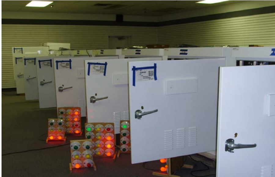
FIGURE 6 Testing of traffic signal controllers and cabinets at the test facility.
