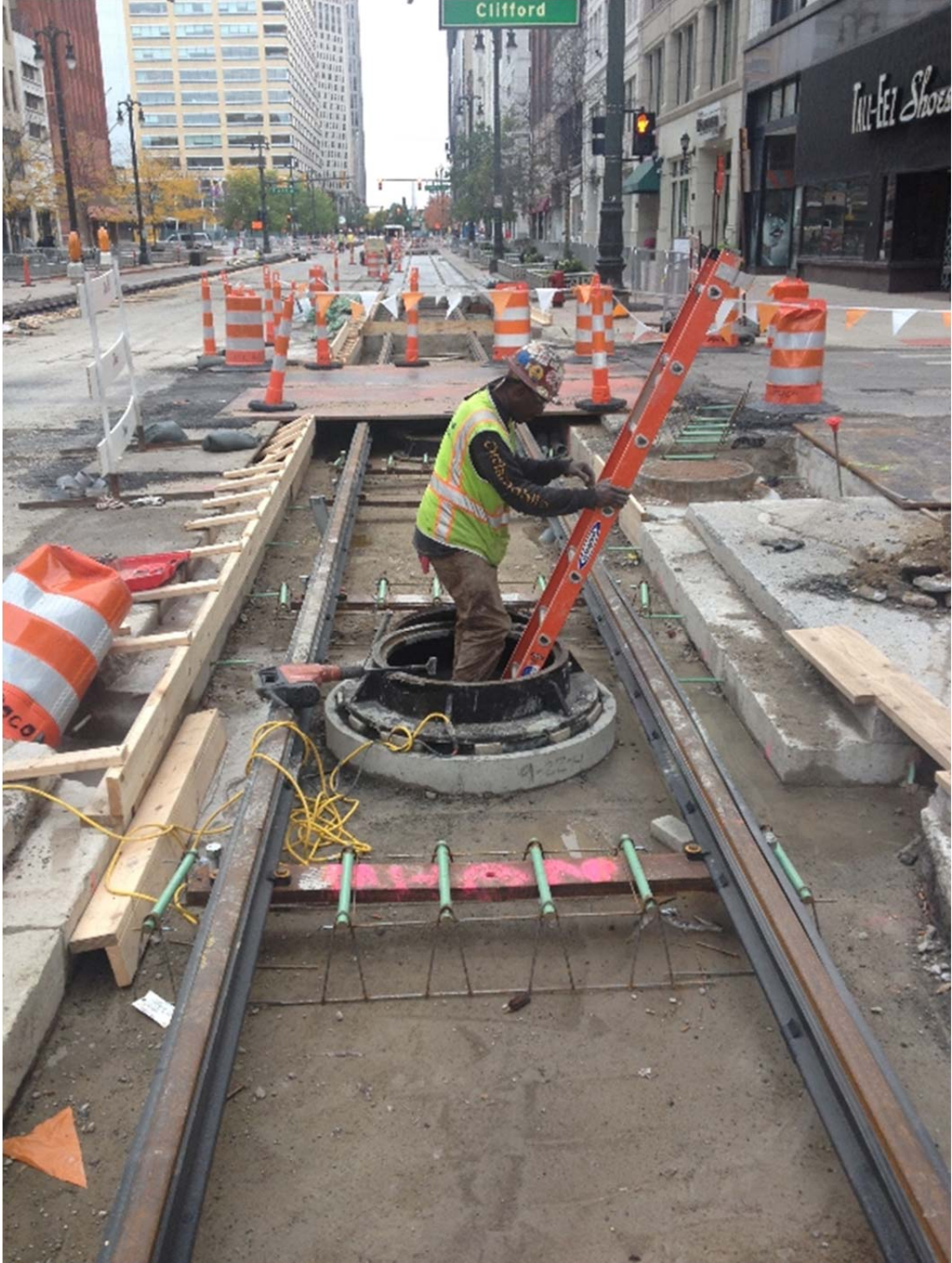
FIGURE 9 Construction of the M-1 RAIL streetcar required reconstruction of streets that had 300 years of utilities and other infrastructure beneath them.
