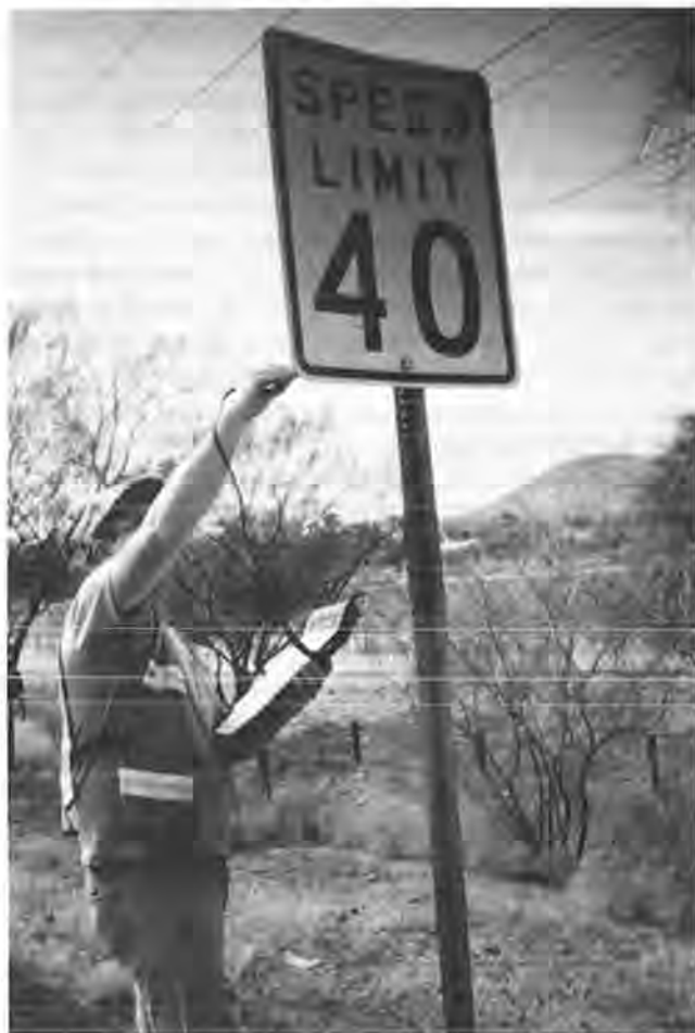
FIGURE 3 Barcoding and pen-based systems are ideal for sign maintenance and inventory management (photograph taken in Arizona).
