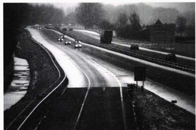
FIGURE 9 Evident difference in behavior of main road and shoulder (porous asphalt) and exit ramp (dense asphalt).
