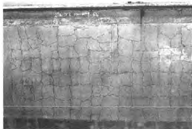
FIGURE 3 Close-up of underside of I-65 bridge at midspan with hairline cracks highlighted.
