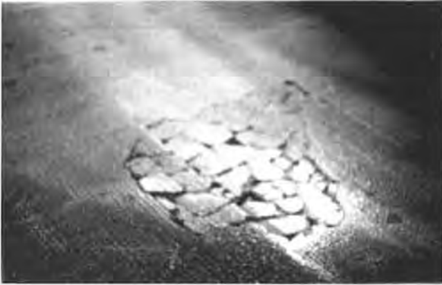
FIGURE 10 Typical deck damage away from joints, Kentucky bridge.
