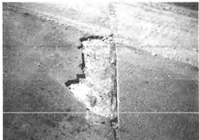
FIGURE 9 Typical deck damage at joints, Kentucky bridge.
