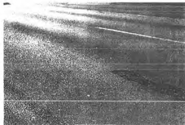
FIGURE 4 I-65 deck surface spall.
