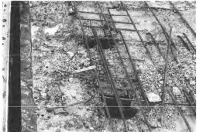
FIGURE 7 Hydrodemolition portion of deck near an expansion joint with two sizable blow-outs—I-285 bridge, Georgia.
