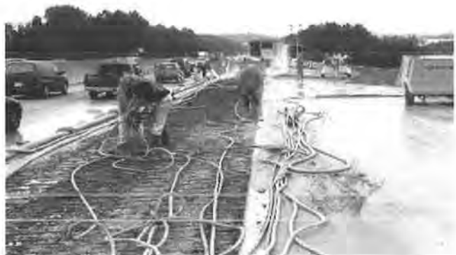
FIGURE 8 Strip to be overlaid just after completion of hydrodemolition looking south on I-285 bridge, Georgia.
