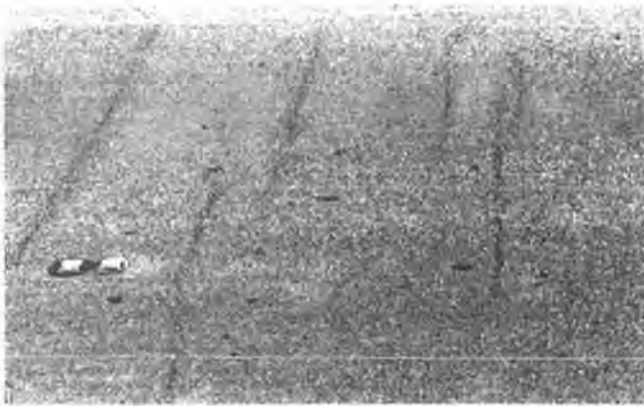
FIGURE 1 Close-up of transverse cracking on I-65 bridge.
