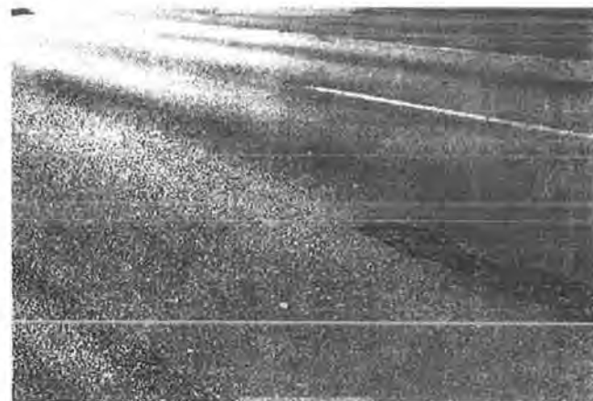
FIGURE 4 I-65 deck surface spall.
