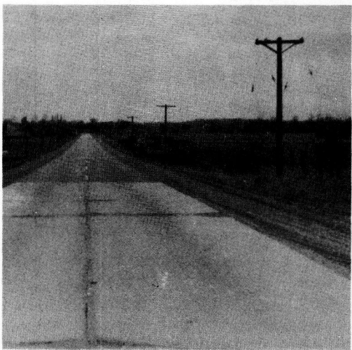
Figure 11. Same pavement as pictured in Figure 10. Pavement in immediate foreground is over Miami soil; bituminous pavement and lift course has been placed over pavement constructed on Clyde soil; pavement has not been covered where it rests on Fox soil. Photo taken in 1954.
