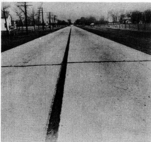
Figure 8. Pavement constructed on Plainfield sand in 1927 without transverse joints - photo taken in 1944 by A. T. Bleck; some transverse cracking at intervals of 120 and 66 feet.
