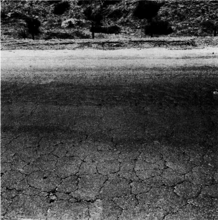
Figure 4. Typical illustration of "chicken wire" or "alligator" cracking.
