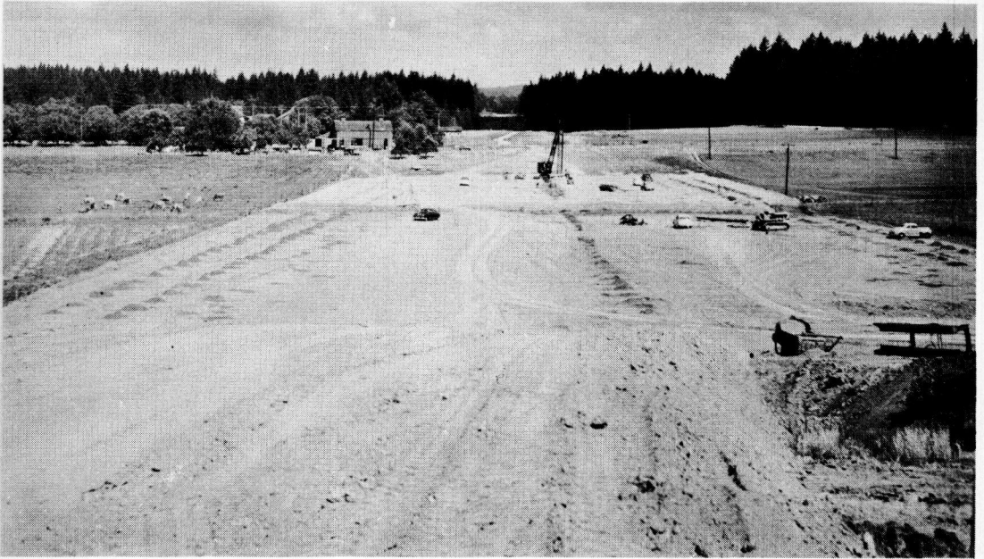
Figure 3. Working platform looking north, summer, 1952. Companion figure to Nos. 15 and 16. Pressure relief drain layout shown by excess \frac{1}{4} in. -0 drain material.
