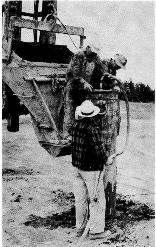
Figure 6. Clamping the air pressure cap on steel mandrel filled with \frac{1}{4} in. -0 drain material. Note the driving cap on the ground lower right.
