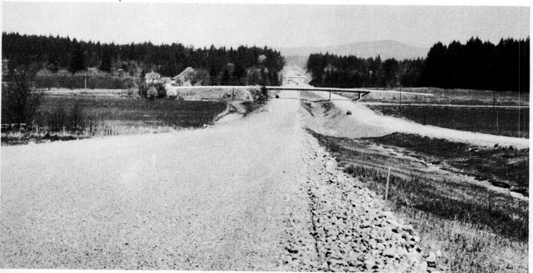
Figure 16. Looking north along west embankment just prior to placing asphaltic concrete paving. See Figures 3 and 15.
