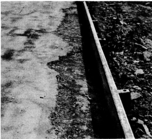
Figure 15. Condition of soil-cement surface along form line caused by blading after mixture hardened. Locations at which this condition occurred were infrequent.
