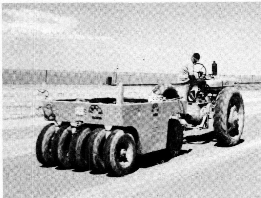
Figure 5, The sandy soil encountered on this soil-cement project required but few tests, using the short-cut test procedures.
