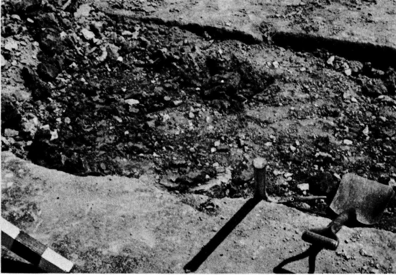
Figure 5. View showing old concrete removed preparatory to patching. This is a minimum width removal of 4 feet.
