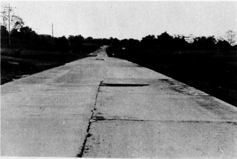
Figure 6. View showing a large size plain concrete patch on left. Right side partially patched. Surface of patches were float finished and were not edged.
