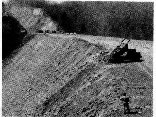
Figure 19. Final stages of end-dumped fill construction. Dressing of fill slopes. Facing west.
