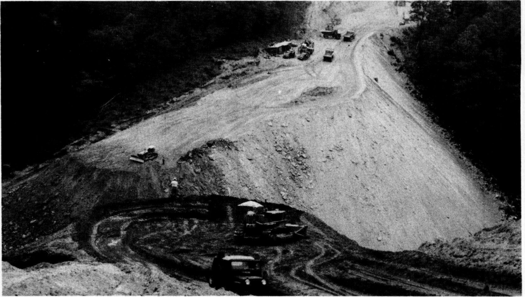
Figure 18. Approaching completion of second ramp. Material is being end-dumped from all sides of fill. Facing east.
