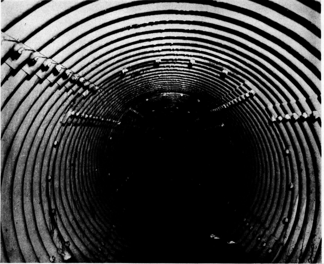
Figure 70. Pipe interior two years after installation.
