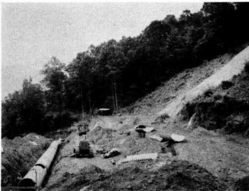
Figure 10. Upward displacement of culvert due to slide action. Facing south.
