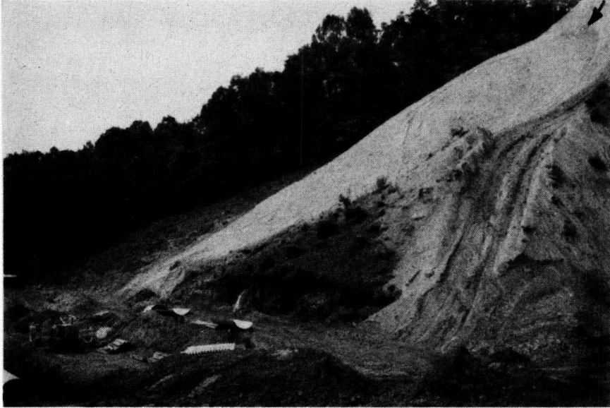
Figure 9. Beginning of slide. Arrow points at trace of failure surface shown clearly on picture.
