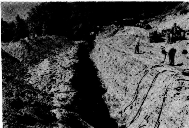
Figure 41. Installation of Ames settlement cells on the compacted fill mass adjacent to the top of the imperfect ditch.
