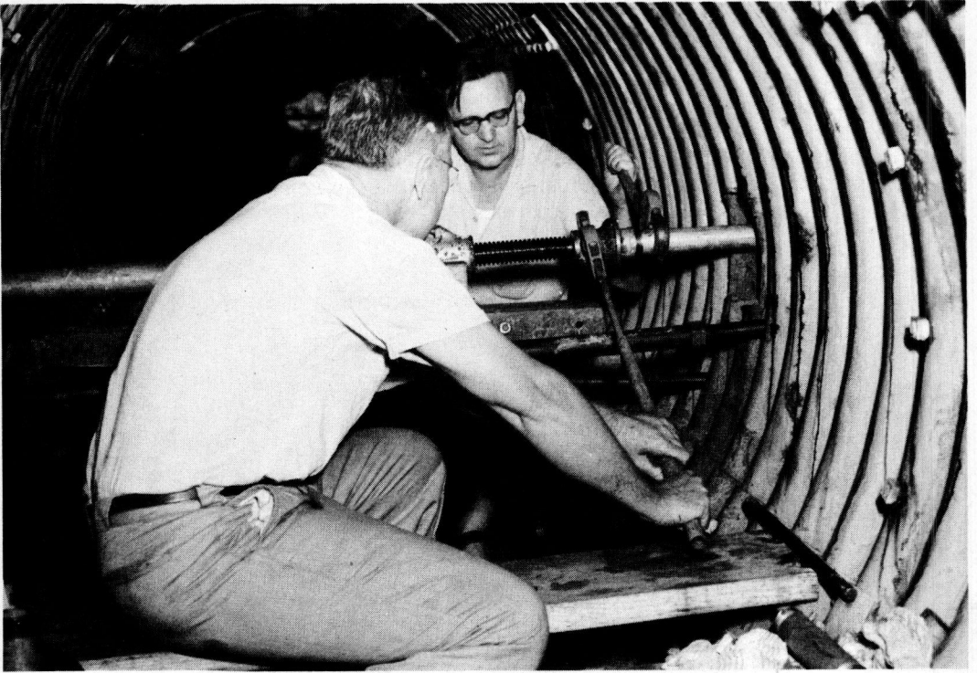
Figure 22. Forcing the sampling device into the side supporting material by means of a mechanical jack.
