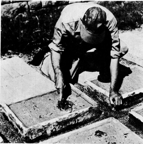
Figure 15. Examination of slabs for scaling.
