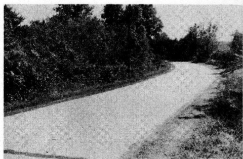
Figure 16 Albemarle County-Scottsville Area Excellent performance of concrete pavement on soil derived from Pre-Cambrian parent material.
