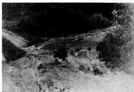
Figure 19 Albemarle County-Scottsville Area A secondary road on soil derived from Triassic parent material. Note poor drainage of plastic soil.
