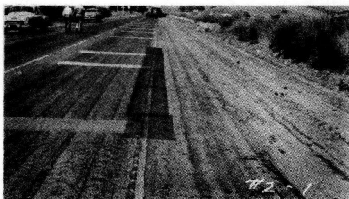
Figure 10. Typical expanded metal test section just prior to paving. Short section of longitudinal joint covered.
