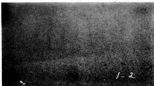
Figure 22. Typical transverse cracking of leveling course following first roller pass. Cracks were closed by traffic within 24 hours.
