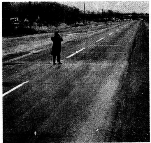
Figure 8. Reflected joints in resurfacing of portland-cement concrete pavement, no base added.
