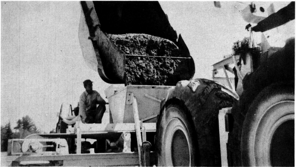
Figure 10. Plattsburg Air Base. Dumpcrete depositing in hopper, (Note "Tourn-a-Dozer" to which belt conveyor is mounted).
