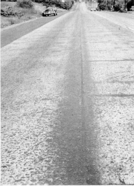
Figure 4. Appearance of joints two weeks after resealing with cold-poured type seal.
