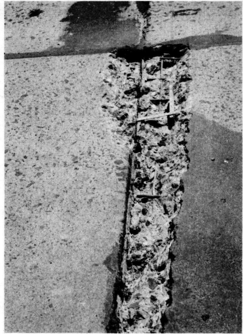
Figure 5. Spalled joint with wire fabric showing.
