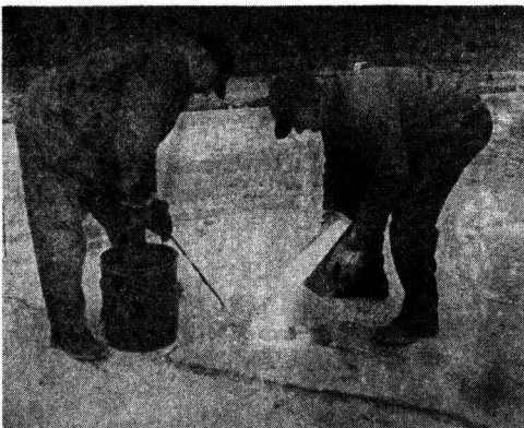
Figure 7. Addition of Calcium Chloride and Water to the Sub-grade of a Highway.
