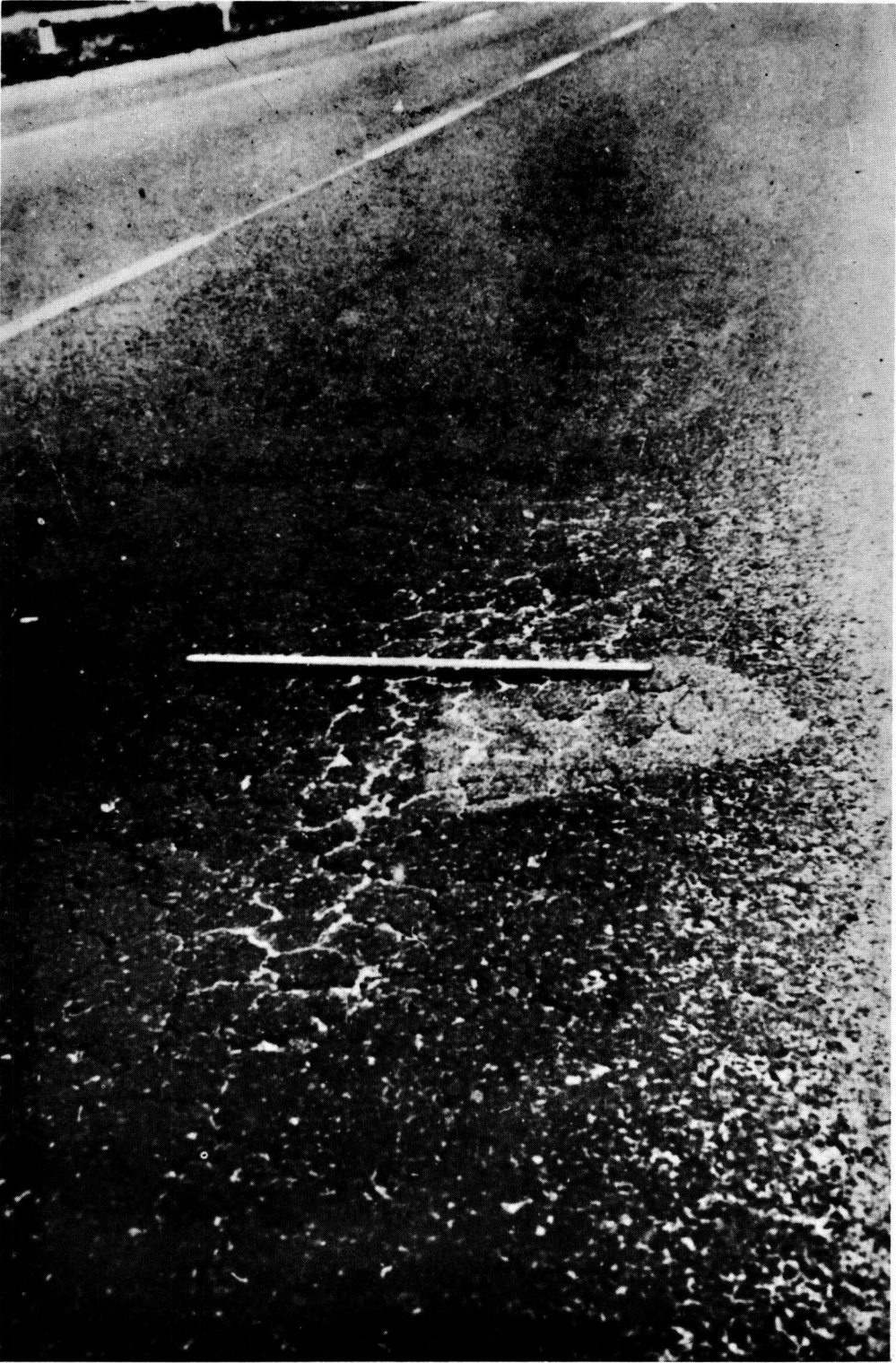
Figure 8. Pavement surface fatigue failure caused by resilient deformations of the subgrade.
