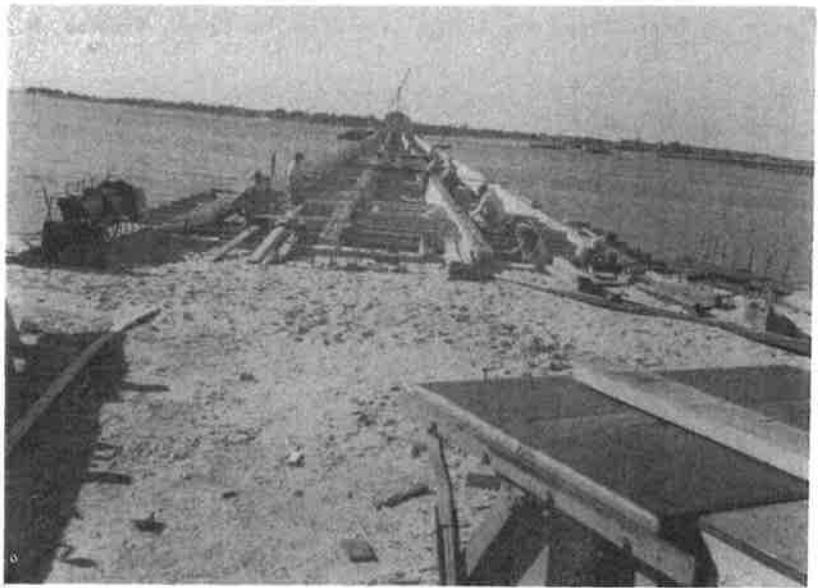
Figure 15. Great Egg Harbor Bay Bridge (looking south). Deck slab forms being erected, Garden State Parkway, N.J.
