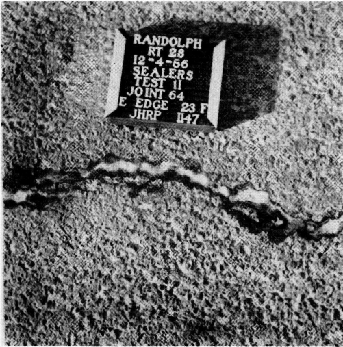
Figure 6. Crack \frac{1}{4} inch or wider with Sealer 1 in good condition.
