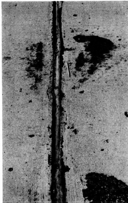
FIGURE 19. ADHESION FAILURE ; TYPICAL OF JOINTS RESEALED WITH BRAND B AT 2 1/2 YEARS.
