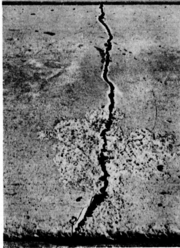
FIGURE 13. SAME CRACK AS IN FIGURE 12 AFTER SEALING.
