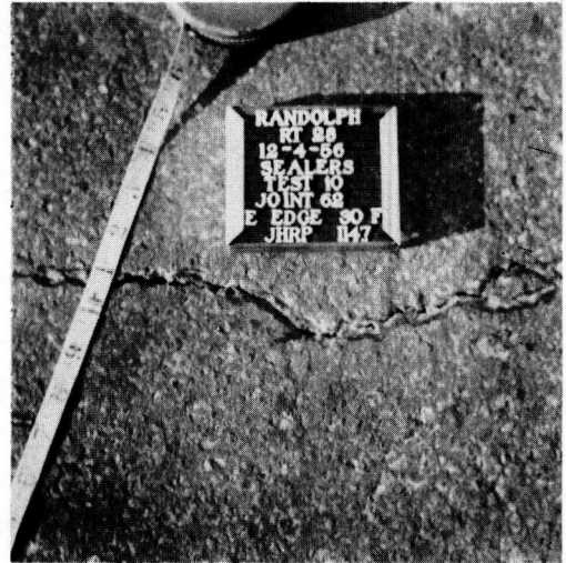
Figure 7. Crack below \frac{1}{4} inch width was not well sealed.
