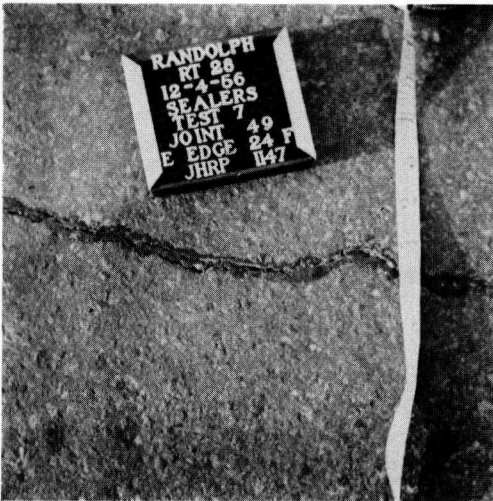
Figure 8. Sealer failed in adhesion.
