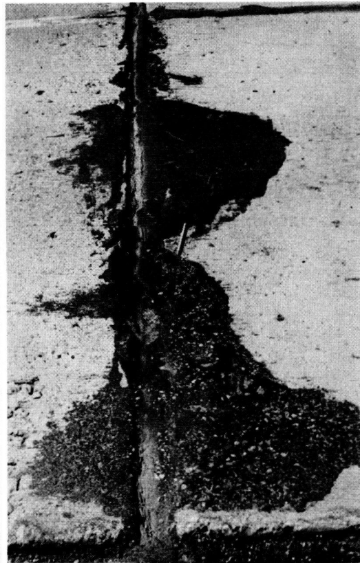
FIGURE 20. SEAL STILL INTACT. TYPICAL OF JOINTS CONTAINING BRAND C AT 2 1/2 YEARS.
