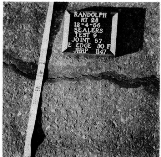
Figure 9. Sealer failed in cohesion.
