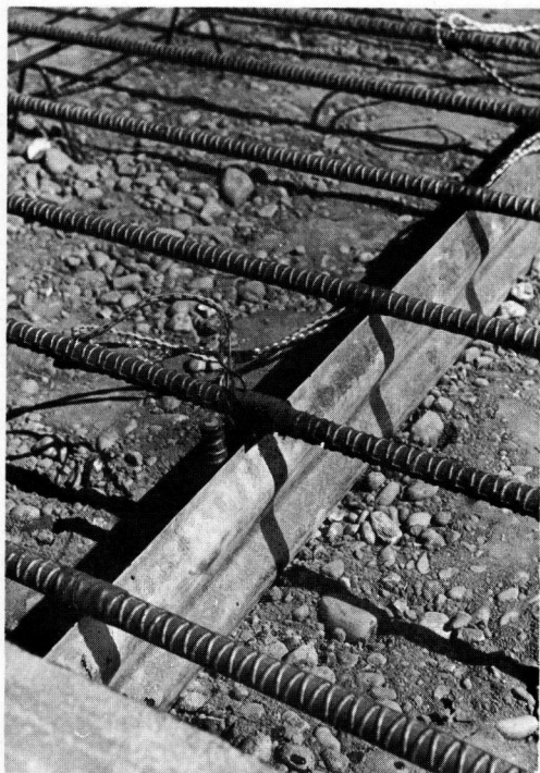
Figure 5. Installed instrumented bar-mat, showing instrumented bars, uninstrumented bars, and crack-former in place.
