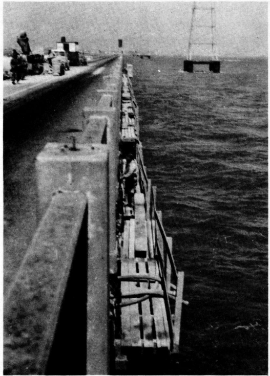
Figure 14. Showing outboard end of Contractor's staging. Each stage spans more than full width of structure deck.
