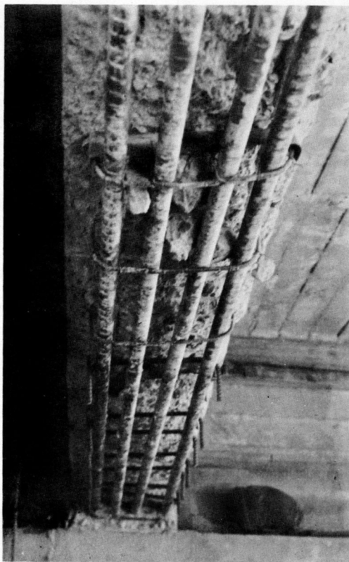
Figure 6. Beam bottom after chipping and before sandblasting, showing spotty and discontinuous areas of corrosion on reinforcement. Stirrup replacements at end of beam yet to be installed.
