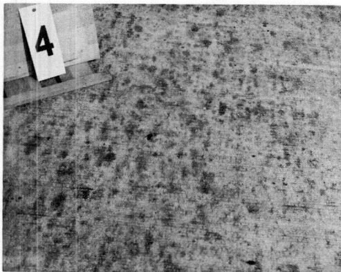
Figure 3. Driving lane of a concrete pavement constructed in 1951 with heavy accumulation of oil droppings on surface.
