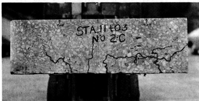
(a) Cracking in base of 14-in. pavement slab after 30,000 coverages of 100 kip twin wheel load traffic.
