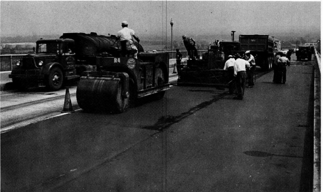
Figure 6. Goethals Bridge, laying silica sand asphalt \frac{1}{2} in. thick using standard asphalt equipment.
