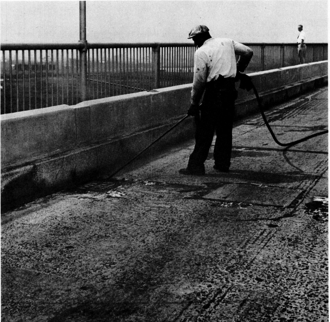
Figure 5. Goethals Bridge, cleaning concrete pavement with compressed air prior to applying tack coat.
