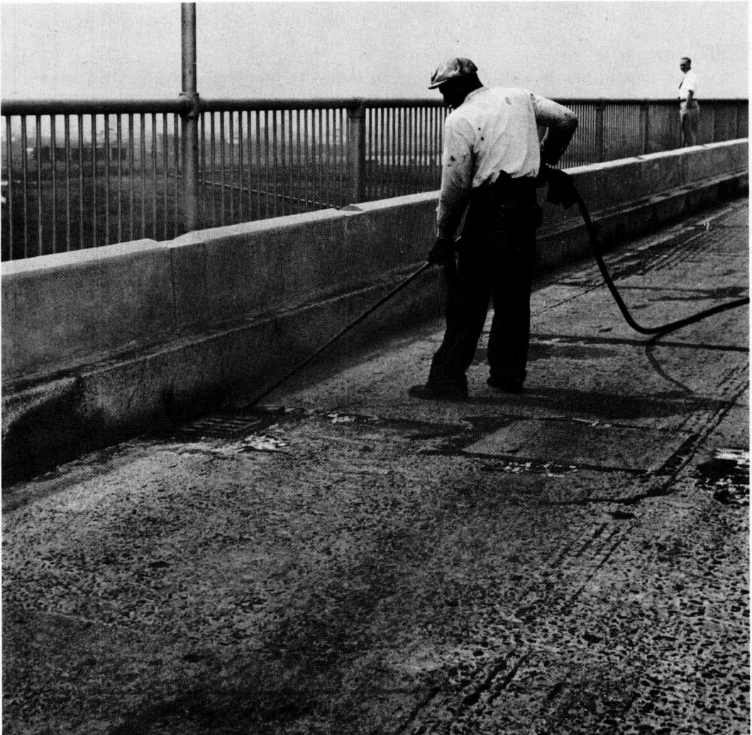
Figure 5. Goethals Bridge, cleaning concrete pavement with compressed air prior to applying tack coat.
