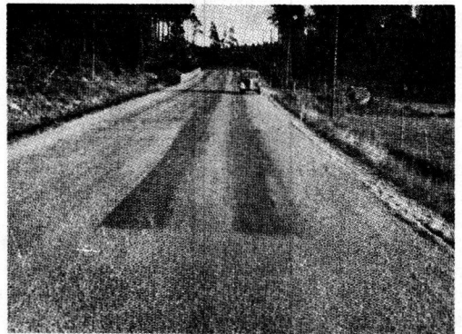
Figure 6. A maintenance seal coat on a Swedish road with cut-back (MC - 5) containing 1.5 percent amine (in foreground) and the same seal coat but without amine (in background). Seal coating was made in good weather—heavy rainfall three days later.
