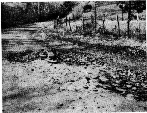
Figure 12. Distress of a Surface Treated Mechanically Stabilized Base Secondary Road - Rt. 609, Culpeper County.
