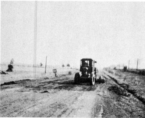
Figure 7. Failure of a Surface Treated Selected Soil Base Road in the Triassic "Red Bed" Soil Area - Rt. 15, Culpeper County - Note typical topography and drainage for this soil area.
