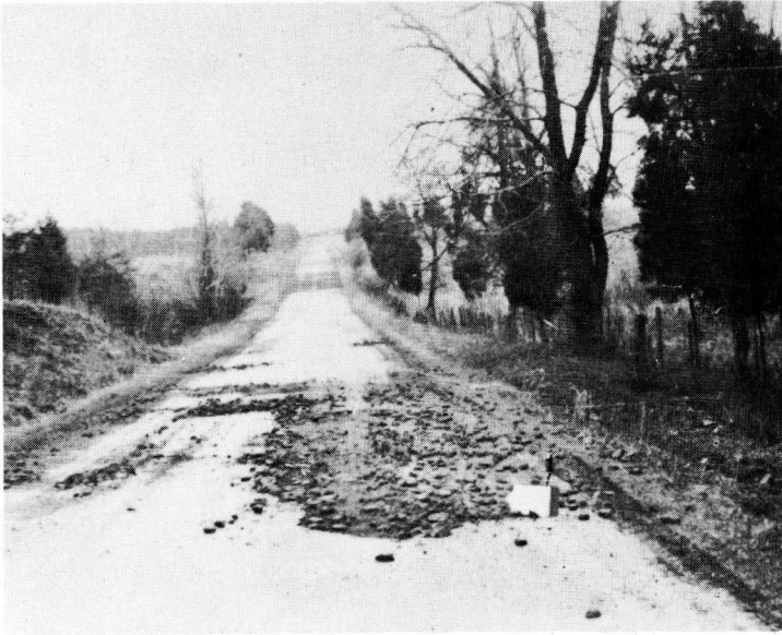
Figure 9. Alligator Cracking and Disintegration of Surface Treated Selected Soil Base Road in High-Quartz Granitoid Soil Area - Rt. 3, Orange County. Because of their high silt content these soils are subject to frost action.
