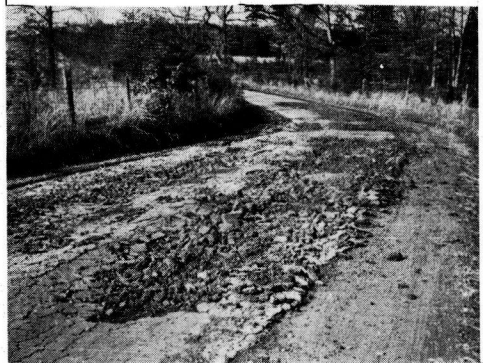
Figure 11. Excellent Performance of a Surface Treated Macadam Base Secondary Road, Rt. 627, Orange County.
