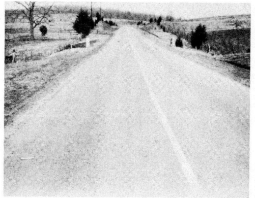
Figure 8. Good Performance of Bituminous Surface Treated Macadam Base in Extrusive Rocks Soil Area - Rt. 15, Orange County.
