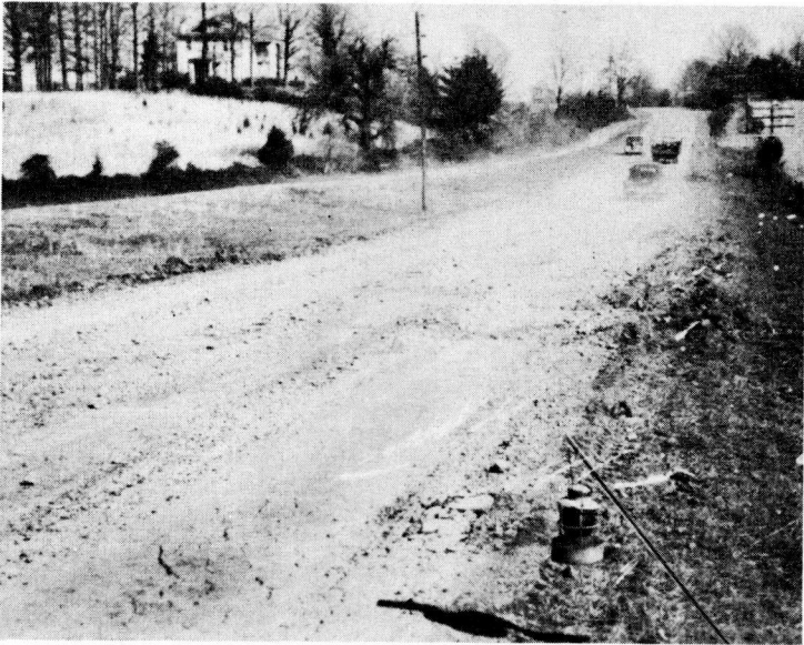
Figure 6. Failure of A Primary Highway (Surface Treated Water-Bound Macadam) - Rt. 29, Culpeper County - This portion of the road is located in Triassic "Red Bed" soil area. Approximately 60 percent of the primary roads in this soil area were rated as poor at the time of the spring break-up.
