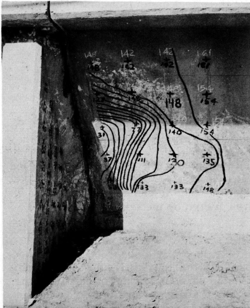
Figure 5. Relative deterioration measured by pulse velocity.
