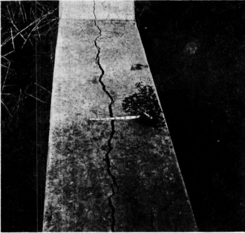
Figure 1. Crack in top face of bridge strut, December 1953.
