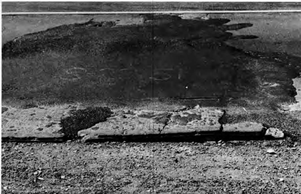
Figure 21. Failure in 10-in. section, Aug. 23, 1951.
