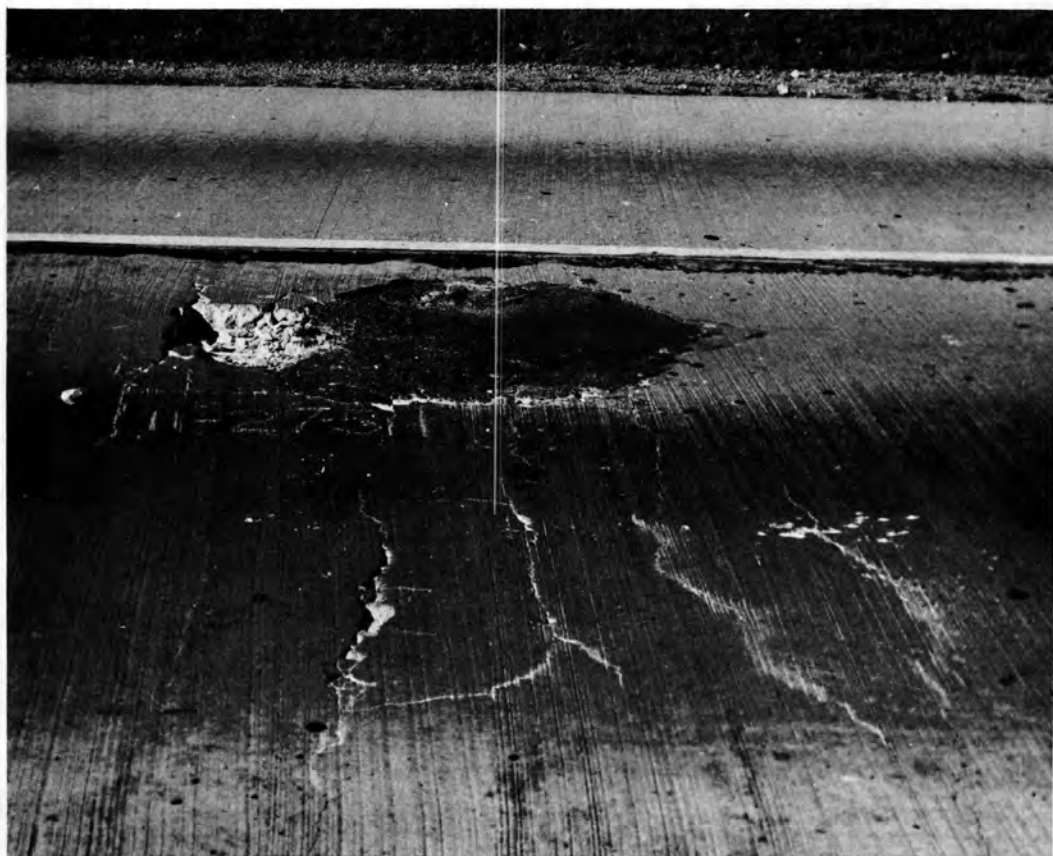
Figure 23. Failed area, 8-in. section, Nov. 27, 1951.
