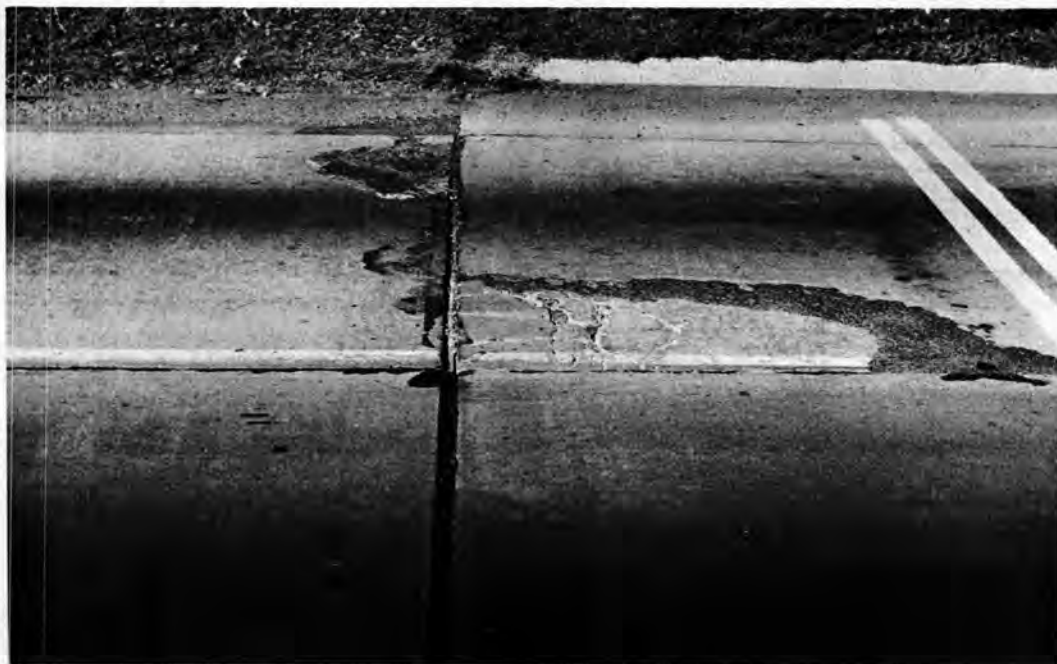
Figure 25. Ruptured terminal joint, 10-in. section, August 1957.
