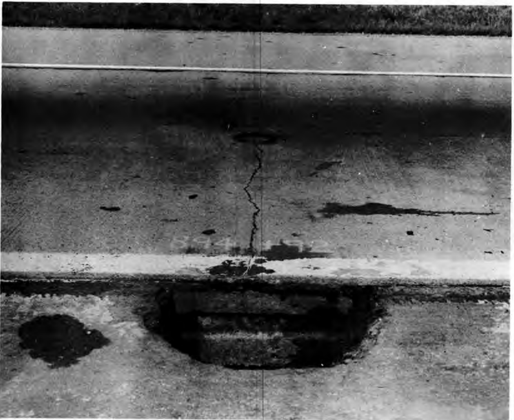
Figure 11. Crack in 10-in. section, Sta. 894+92.
