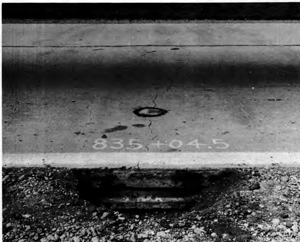
Figure 15. Crack in 8-in. section, Sta. 835+04.5.
