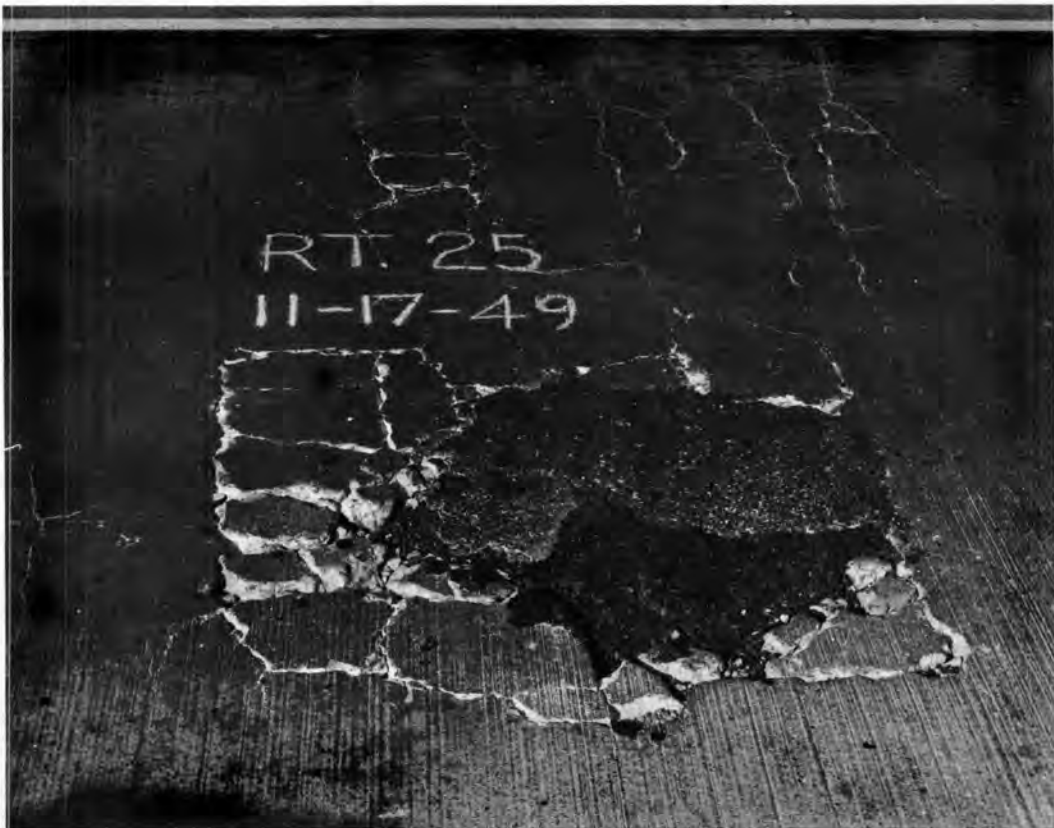
Figure 20. Failure in 10-in. section, Nov. 17, 1949.
