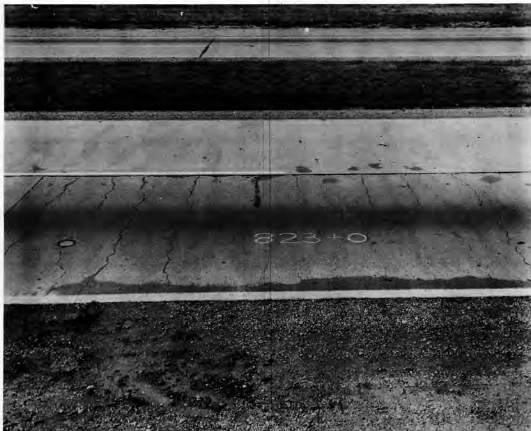
Figure 19. Cracking near construction joint, 8-in. section.
