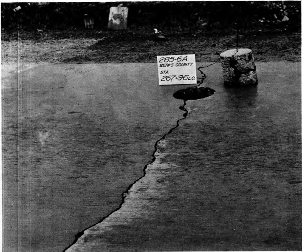
Figure 16. Pavement crack and core at station 267+96.
