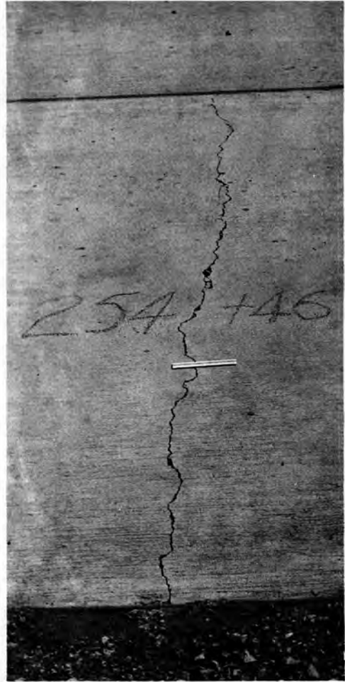
Figure 10. Crack at station 254+46.
