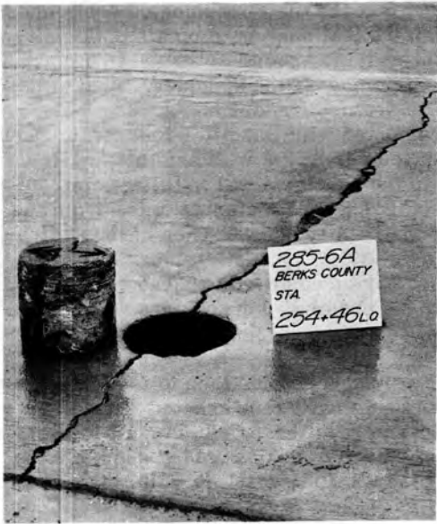
Figure 14. Core from pavement crack at station 254+46.
