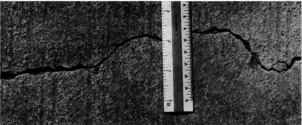
Figure 11. Crack at station 254+46.
