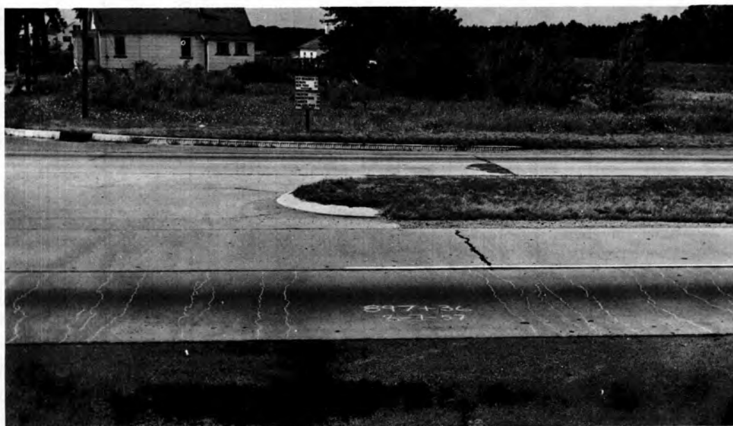
Figure 9. Variable crack spacing, 10-in. section.
