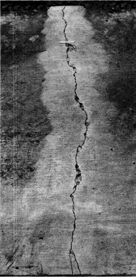
Figure 9. Crack at station 228+85.
