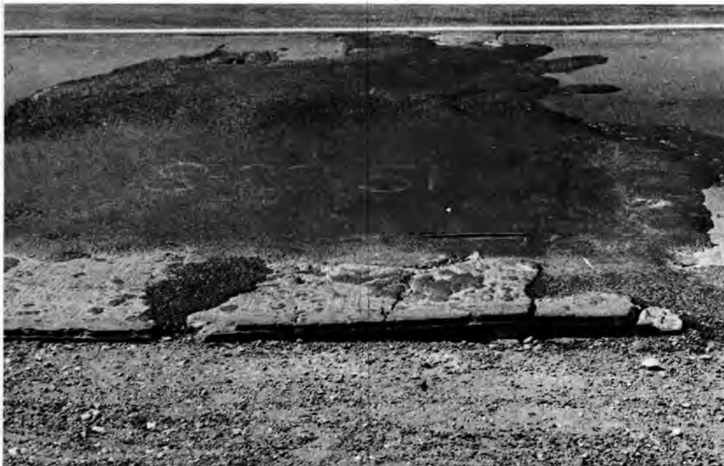
Figure 21. Failure in 10-in. section, Aug. 23, 1951.
