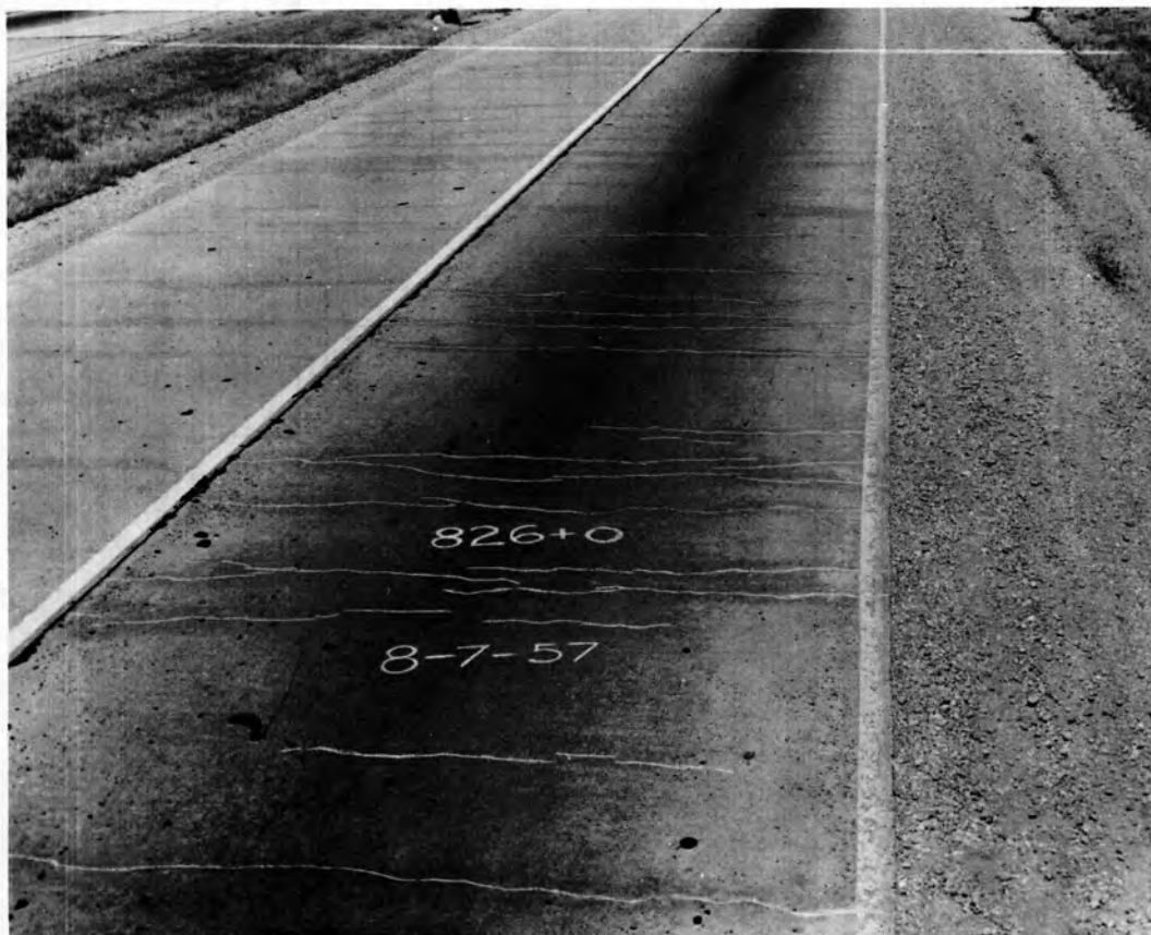
Figure 8. Typical crack pattern, 8-in. section.
