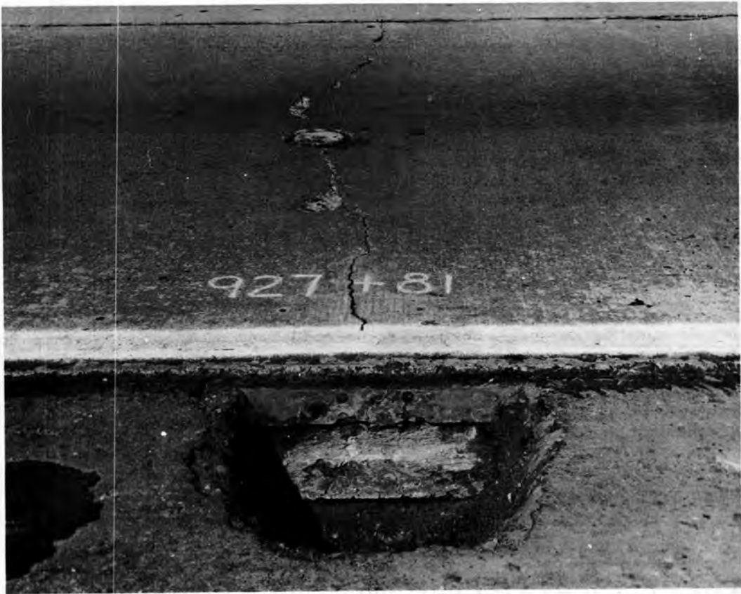
Figure 10. Crack in 10-in. section, Sta. 927+81.
