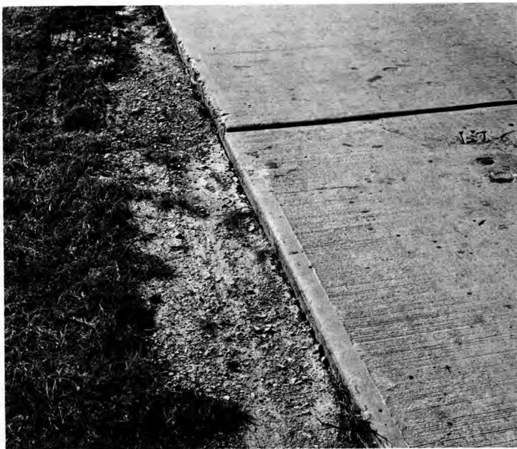
Figure 8. Edge pumping near construction joint in 7-in. pavement with 0.3 percent steel.
