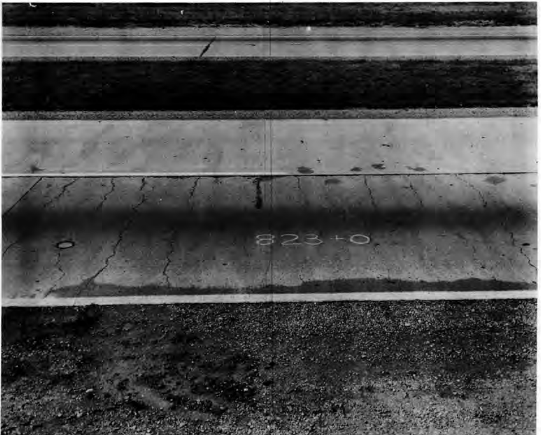
Figure 19. Cracking near construction joint, 8-in. section.
