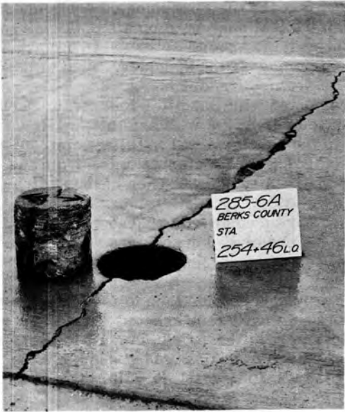
Figure 14. Core from pavement crack at station 254+46.
