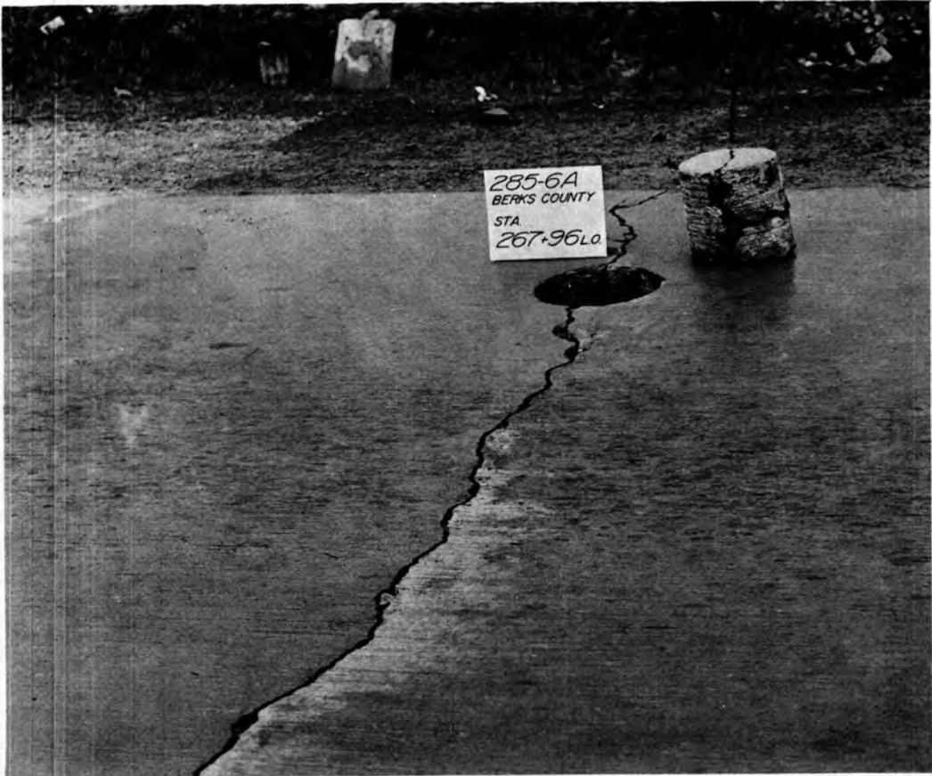
Figure 16. Pavement crack and core at station 267+96.
