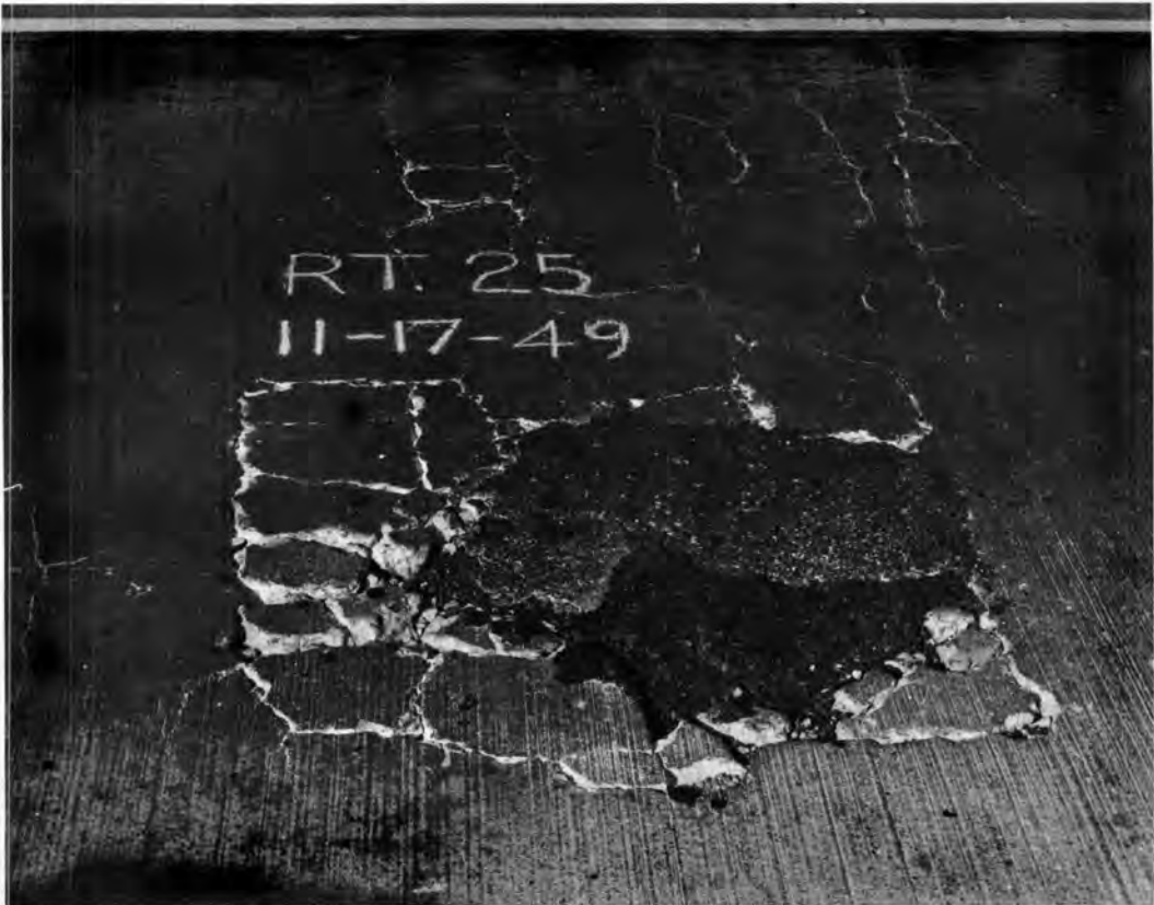
Figure 20. Failure in 10-in. section, Nov. 17, 1949.
