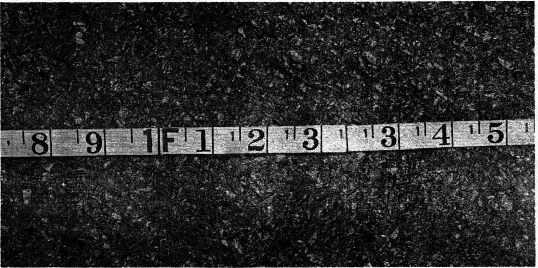
Figure 13. "Poor" site; dense plant-made asphaltic concrete; limestone aggregate, maximum size \frac{1}{2} in., Virginia grading I-3.
