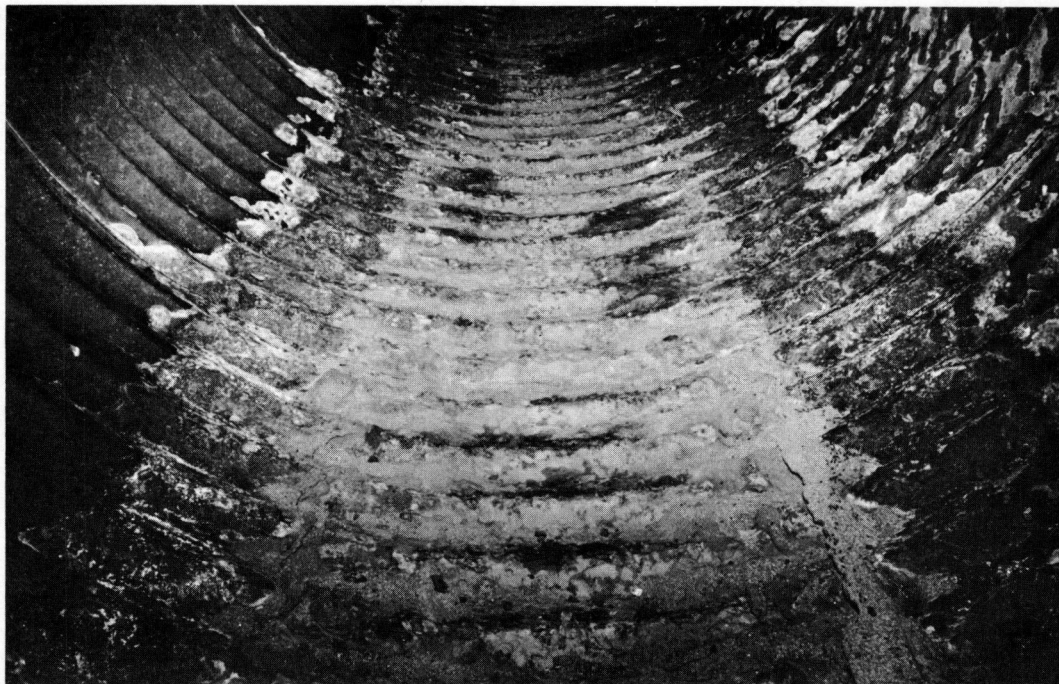
Figure 8. Rusted appearance of a culvert invert as a result of a corrosive flow.
