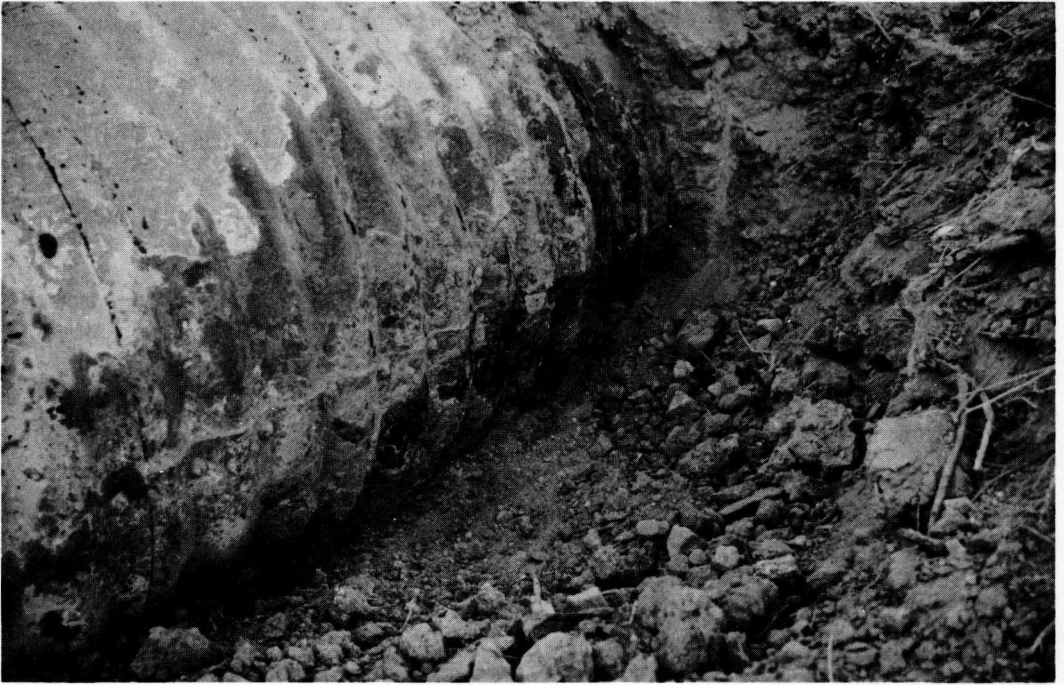
Figure 10. Corroded surface of a pipe contacting a corrosive backfill soil.
