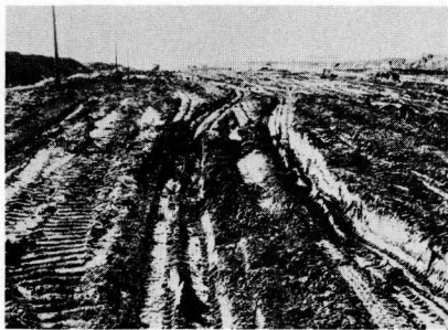
Figure 10. Situation of the job site after rainfalls (untreated soil).
