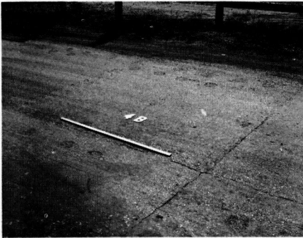
Figure 3. "Satisfactory" performance of dense-graded mix showing no cracking or flushing.
