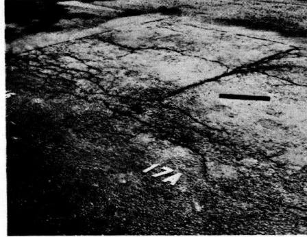
Figure 2. Extensive cracking, characteristic of "brittle" performance.
