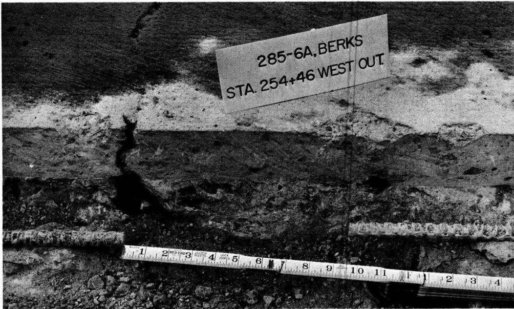
Figure 8. Gap in reinforcing bars.
