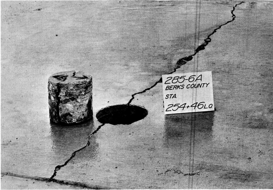
Figure 7. Typical wide crack.
