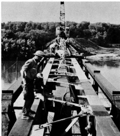
Figure 4. Some of the test areas on protection of top flanges, Chicago Great Western Rwy., Byron, Illinois.
