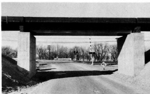
Figure 3. Proprietary paints in relatively sheltered location on rolled beam deck spans. (One of 3 test bridges near Kansas City.)
