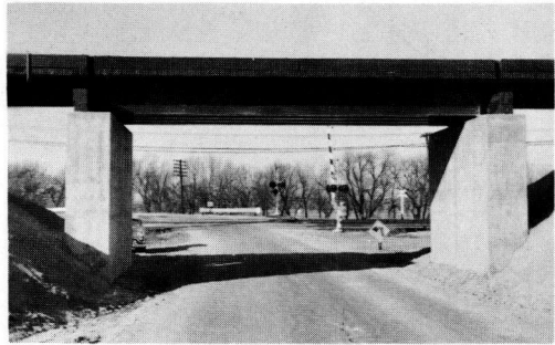
Figure 3. Proprietary paints in relatively sheltered location on rolled beam deck spans. (One of 3 test bridges near Kansas City.)
