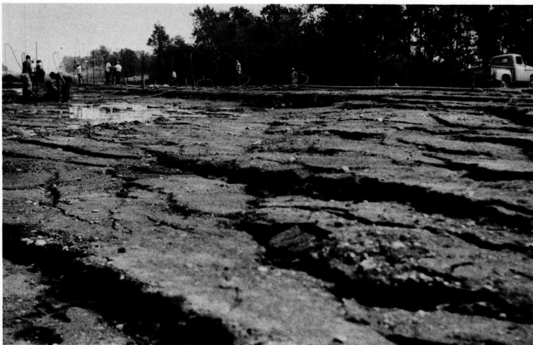
Figure 2. Extensive settlement cracking.
