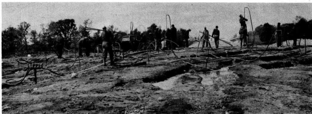
Figure 3. Settlement cracking and jet spacing.
