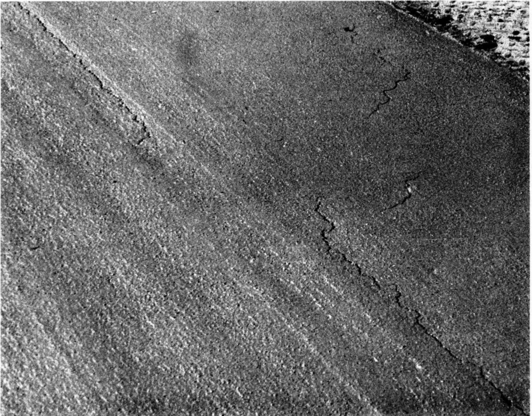
Figure 9. Shrinkage cracks in latex-mortar surface on west end of Lane D when not quickly covered with wet burlap.
