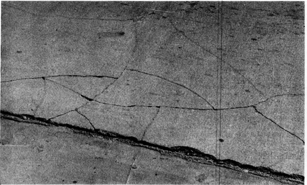
Figure 10. Extensive cracking and loose latex mortar on east end of Lane F after one winter (April 1958).
