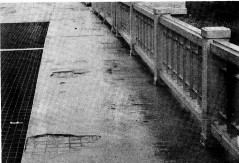
Figure 13. Newly spalled areas in north sidewalk, some adjacent to patches.
