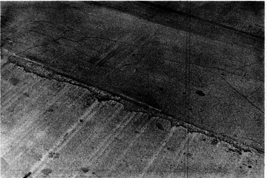
Figure 11. Cracking and loose mortar in west end of Lane D after one winter (April 1958).
