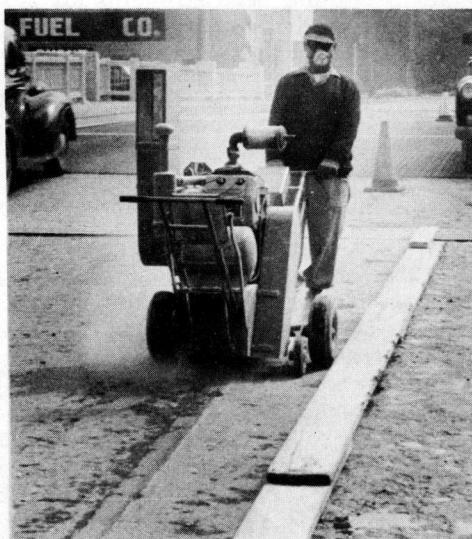
Figure 4. Cutting machine used to remove minimum of \frac{1}{2} in. of scaled concrete.
