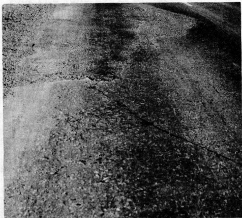
Figure 3. Base failure areas of Milhaven-Swartz road.
