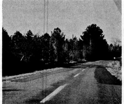
Figure 2. Surface failures and good maintenance work done on patching Sykes-Grayson road.
