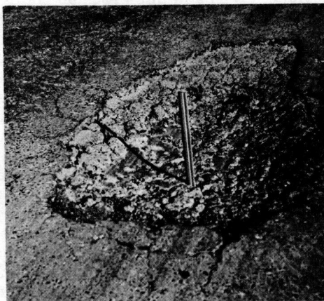
Figure 4. Base failure on Oak Grove-Lake Providence road.
