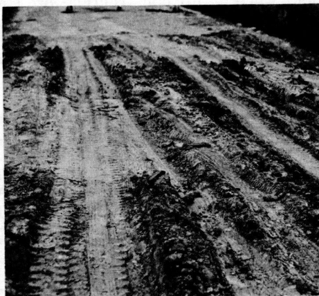
Figure 6. Condition of Highway 14 at Holmwood during the winter of 1958.
