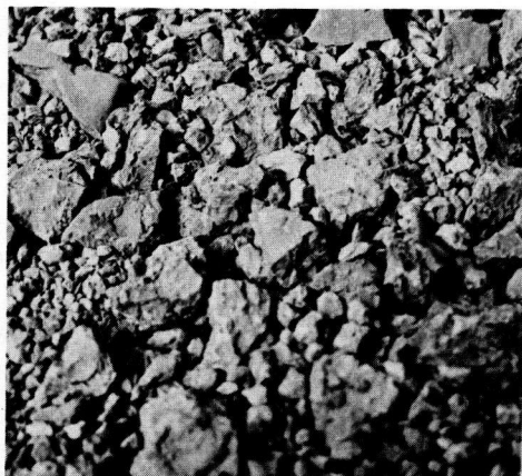
Figure 10. Uniformly mixed and pulverized material after the first application of the lime.
