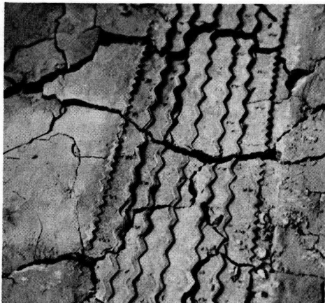
Figure 8. Shrinkage cracks developed on the base before treatment with lime.
