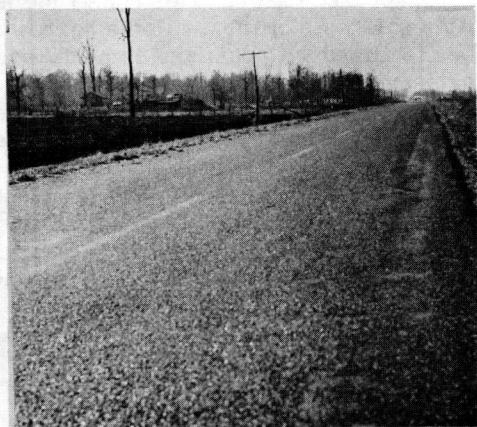
Figure 5. Condition of the Newellton road after two years of service.
