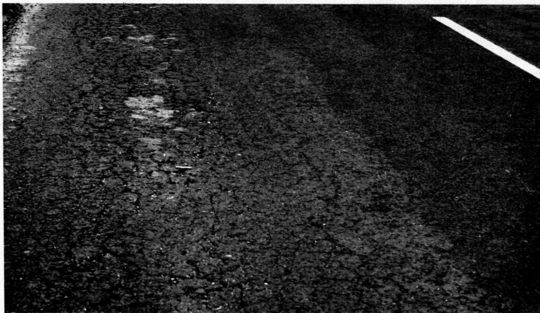
Figure 2. Cracking of pavement described in Figure 1.
